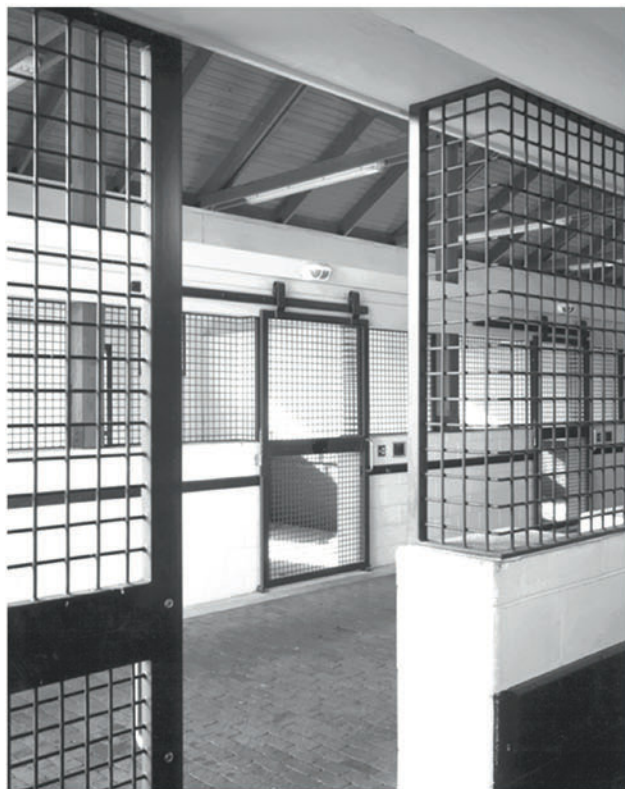
Stall doors of 2 x 2-inch steel mesh maximize air movement. Note the smooth rounded edges on the heavy mesh and block wall beneath it. These stall doors are anchored top and bottom, so that dangerous openings are not created when horses lean against them or push against them with their noses.
